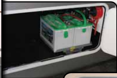
Four compartment battery storage.
